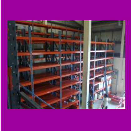
Warehouse Storage Rack
